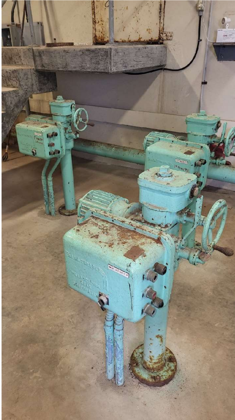
Photograph #14: Valve House Actuator Motor
