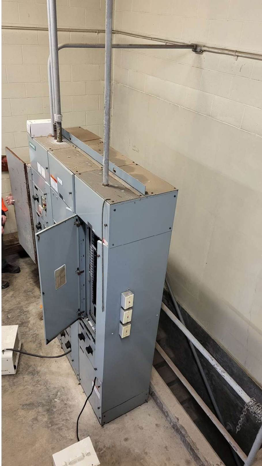
Photograph #3: Top View of Existing MCC in Valve House
