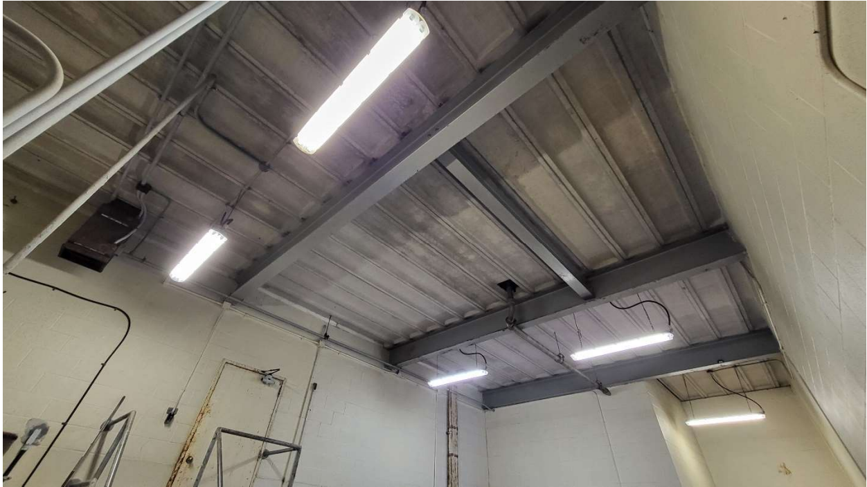
Photograph #8: Valve House Ceiling
