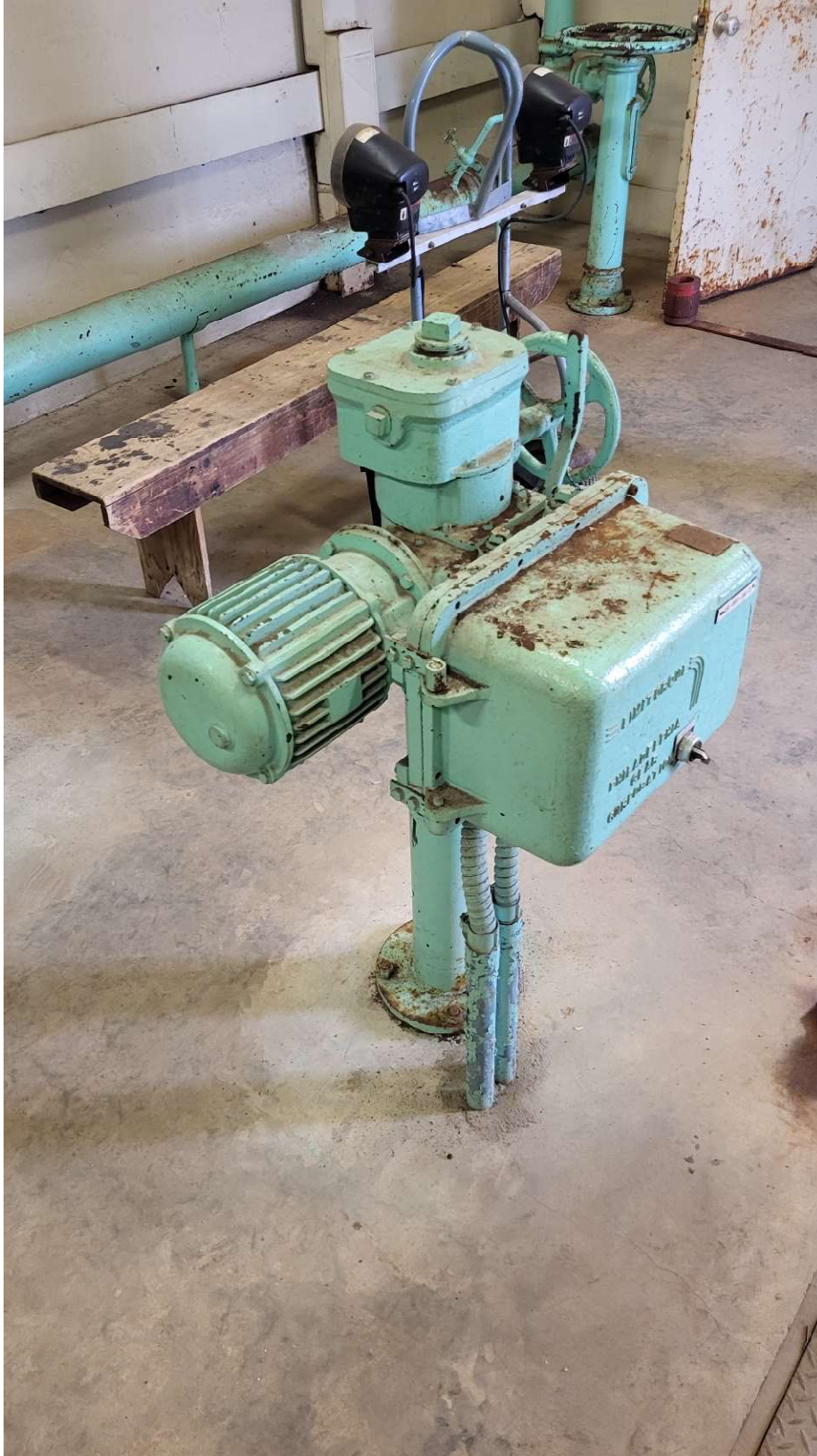
Photograph #16: Valve House Actuator Motor
