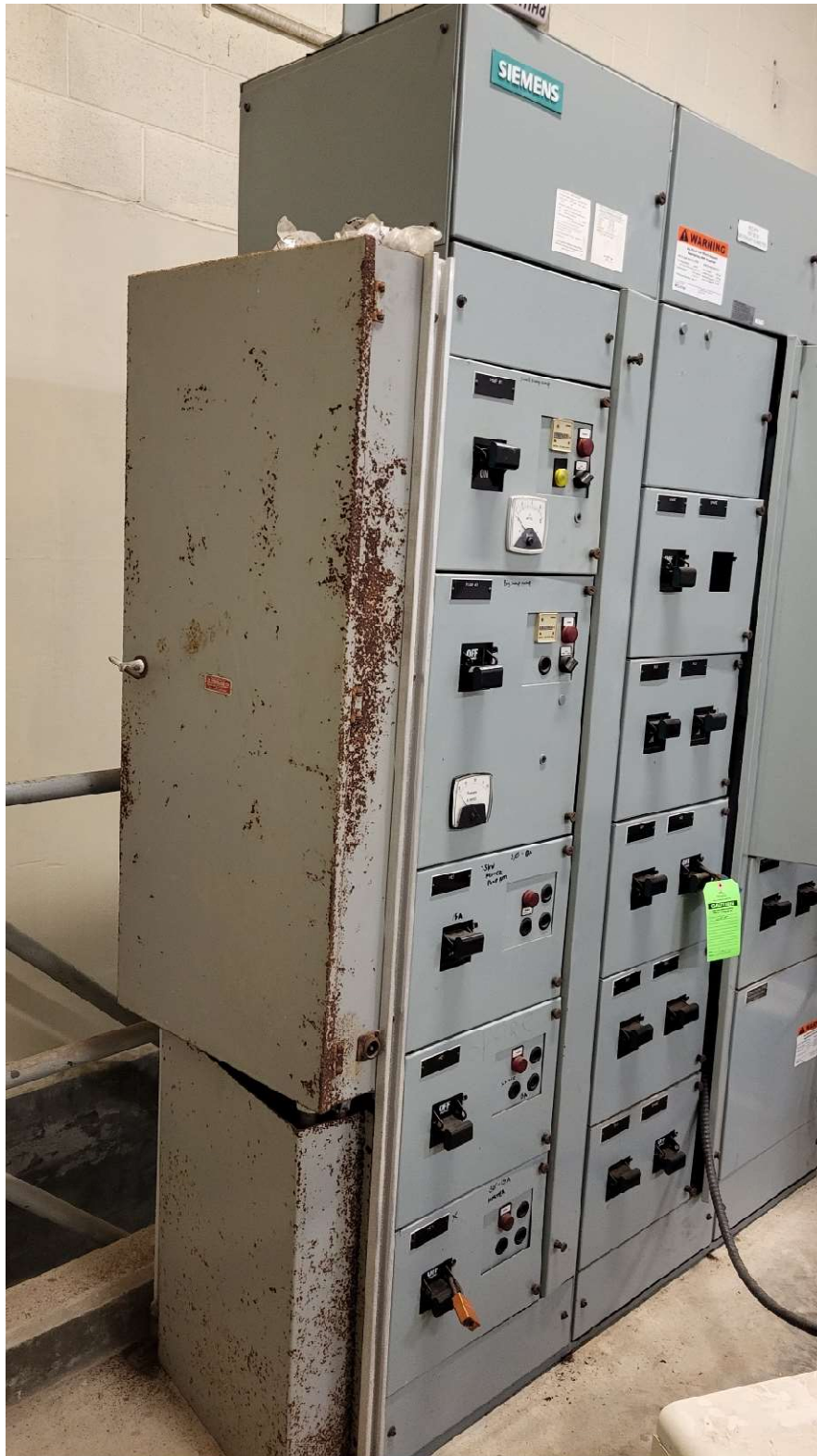
Photograph #1: Existing MCC & terminal Cabinet in the Valve house,
