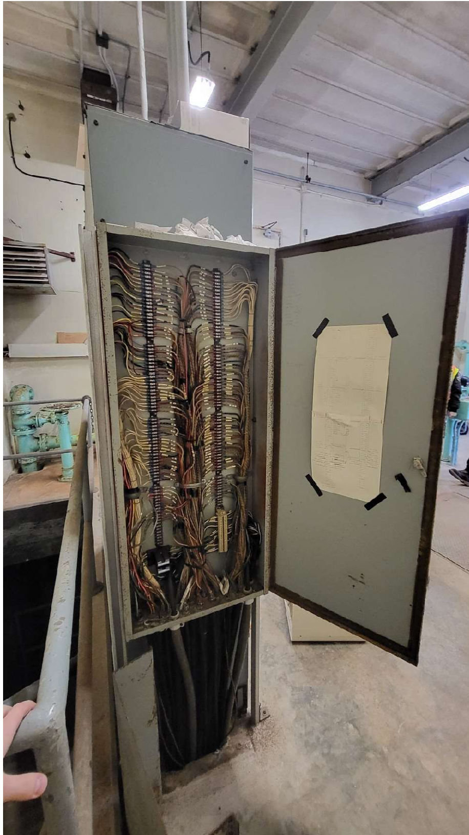
Photograph #5: Valve House Terminal Cabinet
