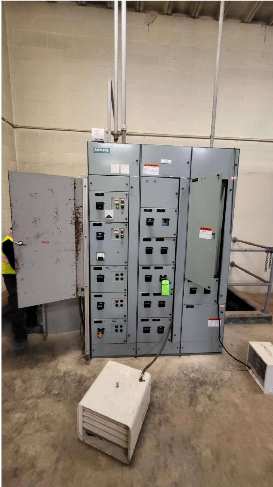
Photograph #4: Existing MCC in Maclean valve house, and temporary unit heater on the ground.
