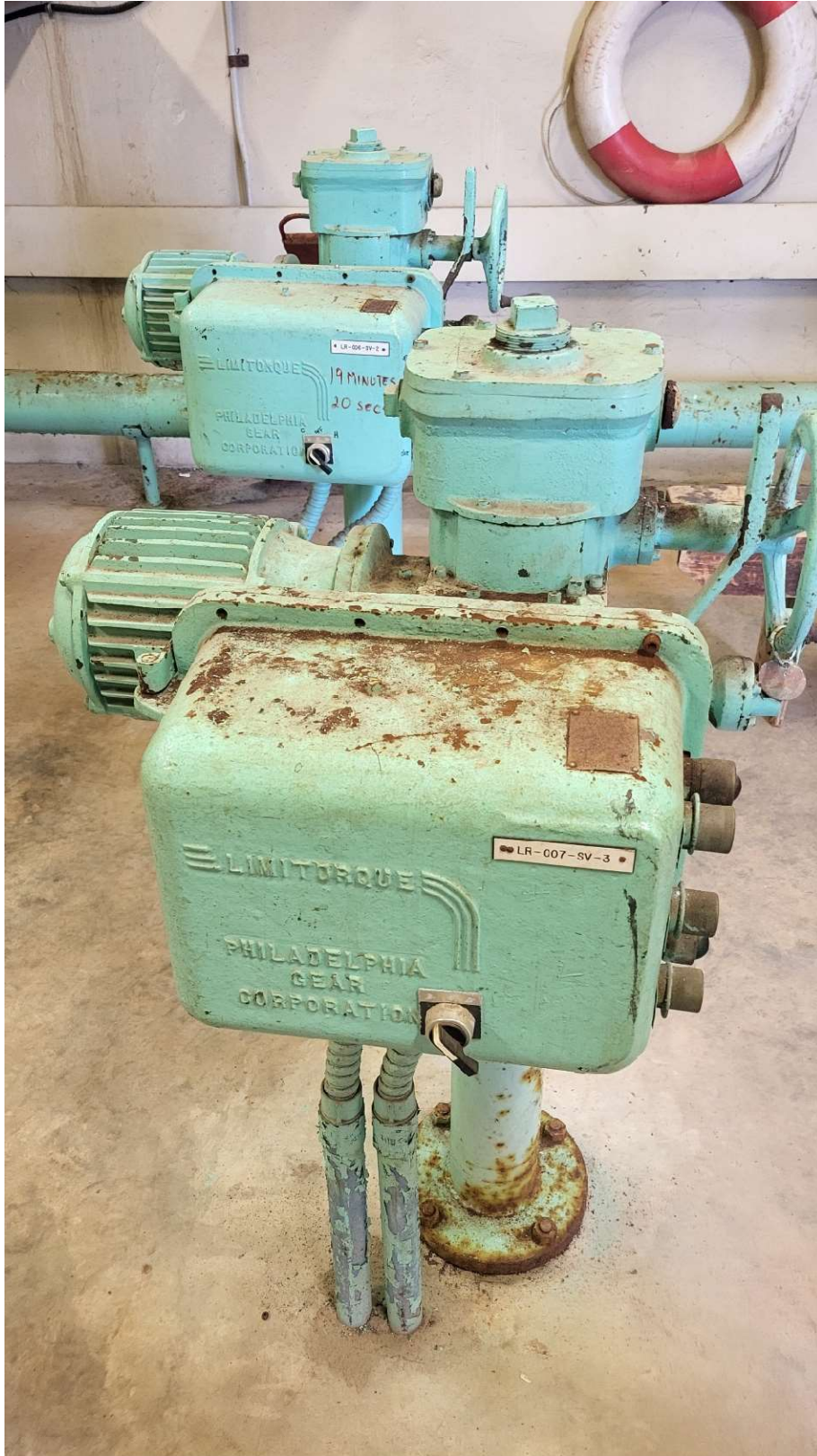
Photograph #15: Valve House Actuator Motor
