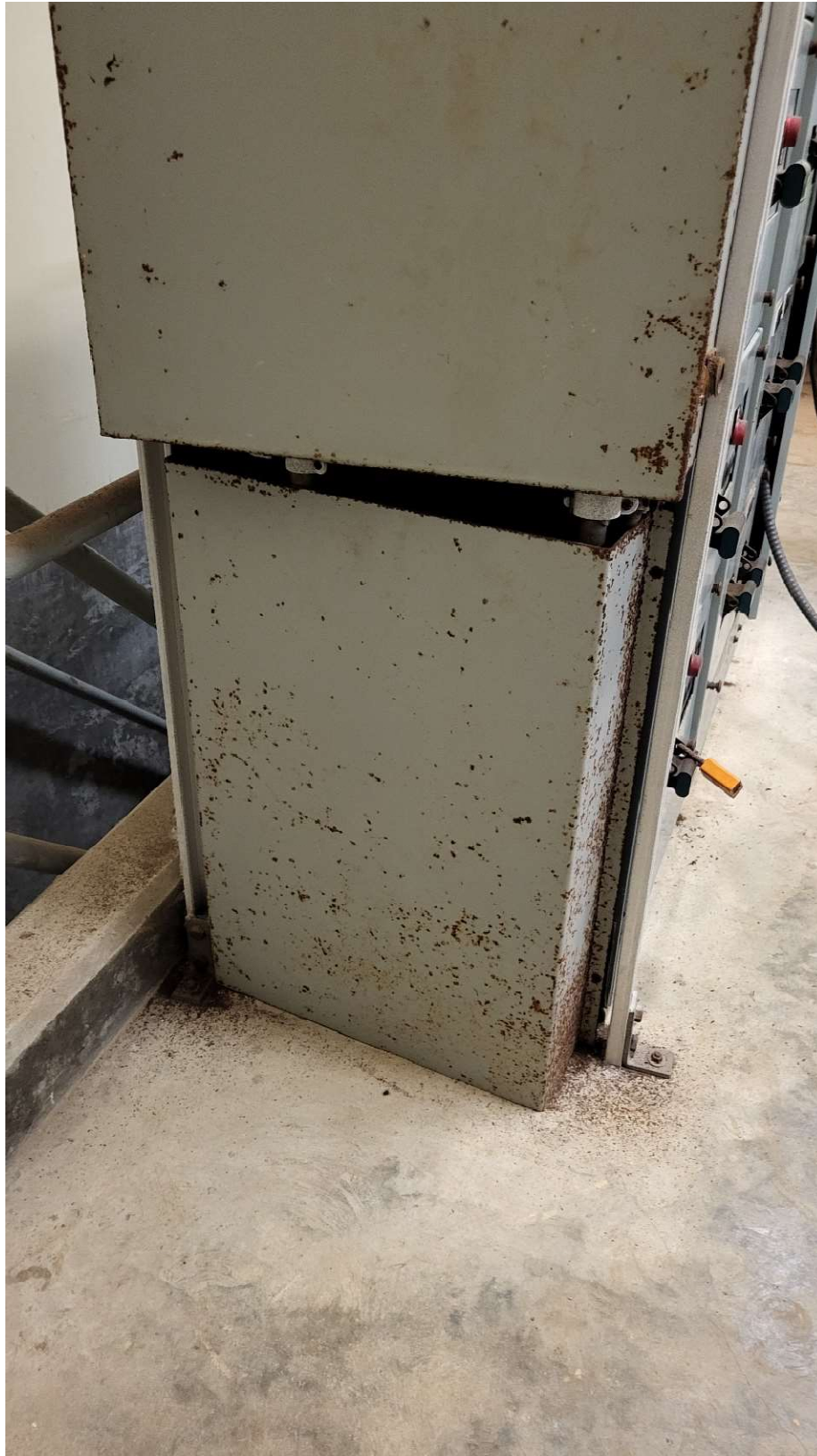
Photograph #2: Valve House Terminal Cabinet
