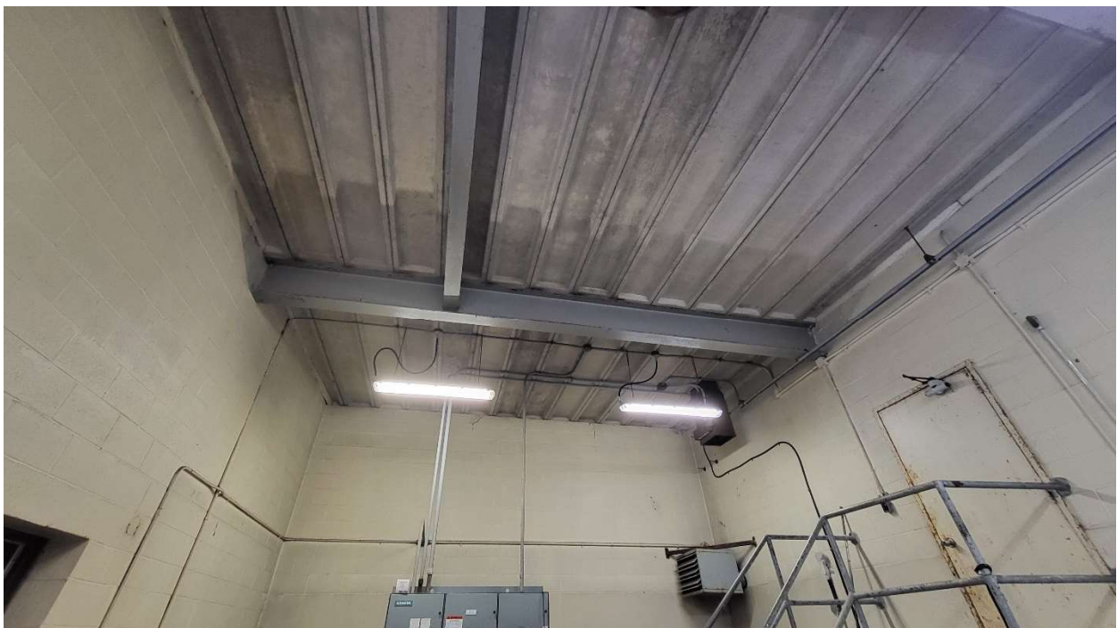
Photograph #9: Valve House Ceiling
